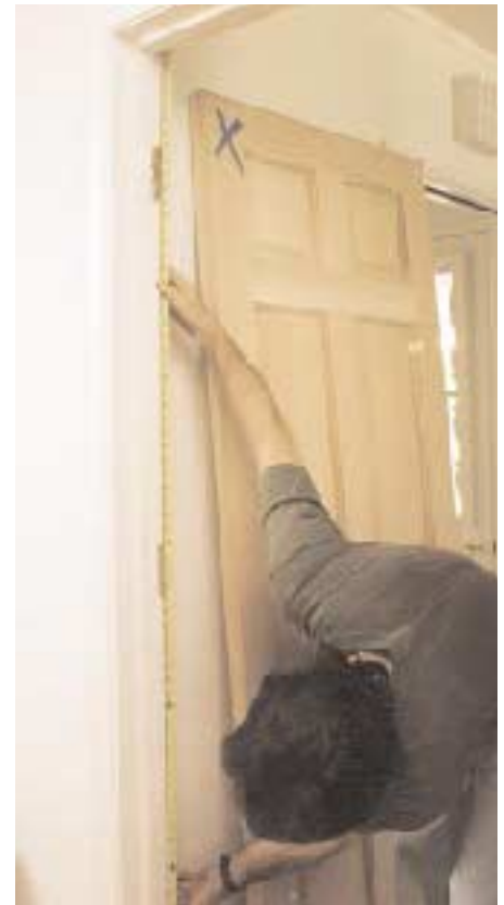
Figure 2. Measure to locate the top of the existing hinges and write the dimensions lightly on the door. To reduce math errors, the author prefers to leave a gap between the tape and the head jamb rather than holding the tape tight to the jamb and subtracting \frac{1}{8} inch.
