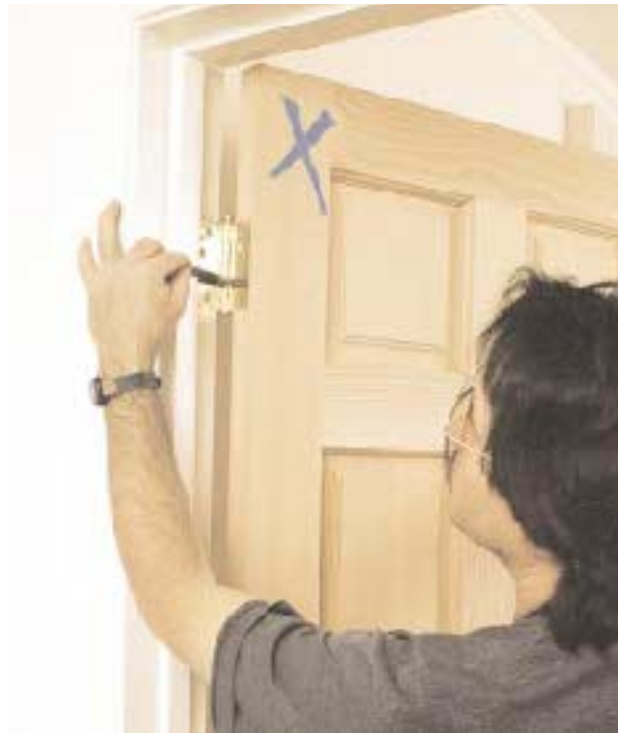
Figure 8. To rotate the door away from the hinge jamb, spread the top or bottom hinge by gently closing the door while holding a nail set between the leaves of the hinge (left). To pull the door toward the hinge jamb, bend the knuckles of the hinge one at a time toward the jamb using a crescent wrench (below).
